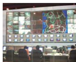
Traffic control center
